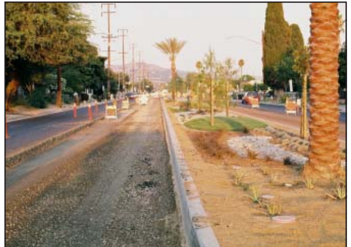
Up to 8 inches and more of asphalt was removed from Beverly Blvd., but only 2 inches or less could have been removed using an ARAM Composite Layering System
