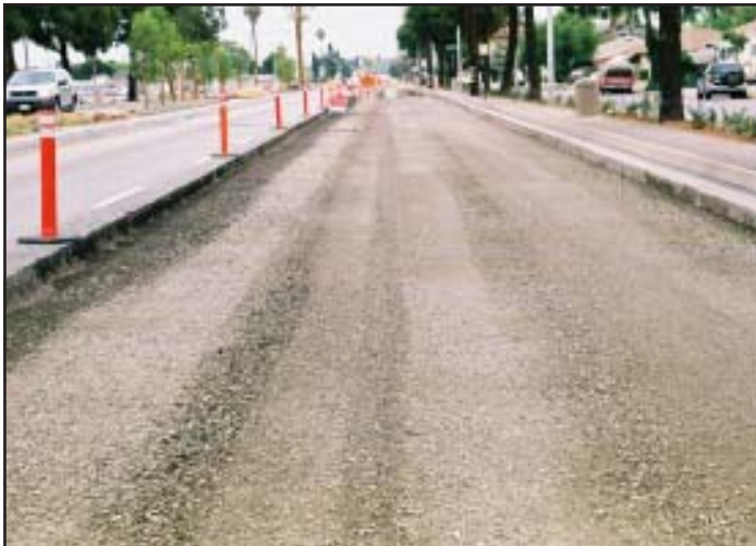
Sections of Beverly Blvd. in Pico Rivera were reconstructed in Summer 2011. This was a perfect candidate for a much more cost effective ARAM Composite Layering System
